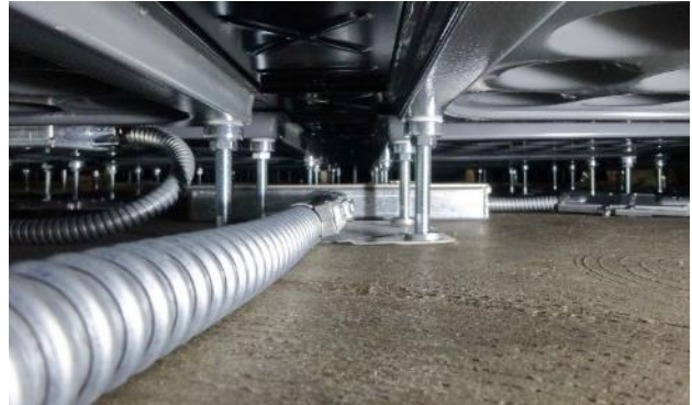
Jumpers connect zone boxes, floor boxes under access floor.
